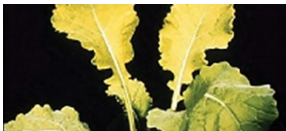
Iron Chlorosis in Canola that can be corrected by adding FeRRoGREEN into the starter.
